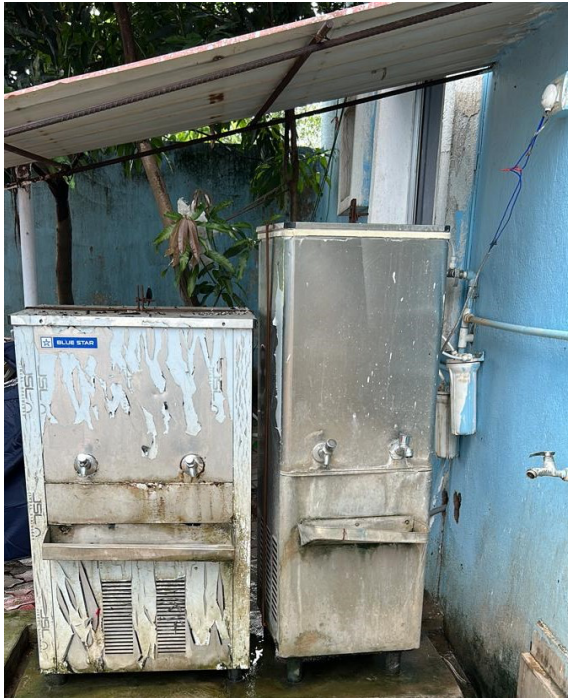
RO Water Cooler – Boys Hostel
